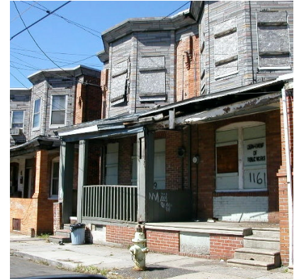
Image 5. Vacant properties which are a blighting influence and represent a health and safety hazard will be acquired.
